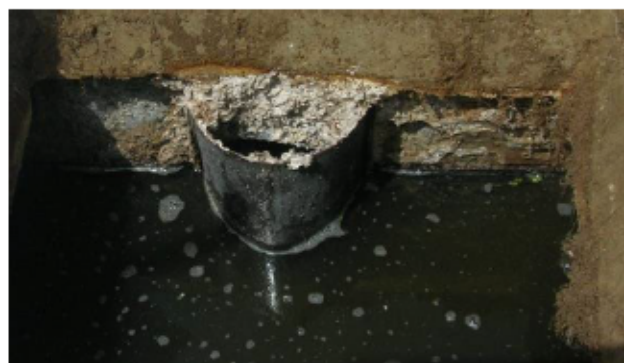
Photo 1 Concrete Corrosion around Outlet Baffle
