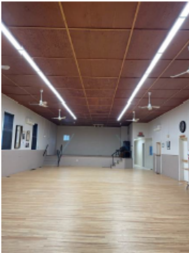
Photo 1. Maberly Hall, LED Lighting
