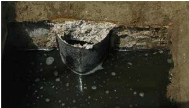
Photo 1 Concrete Corrosion around Outlet Baffle
